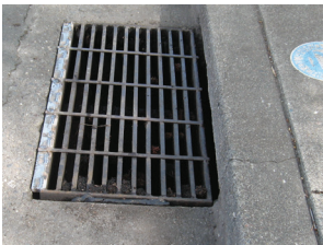
Storm drop inlet, grate
